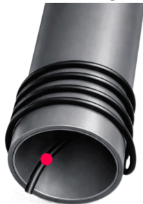
Figure 18 Wrapping of the heating cable around the end of the drain
