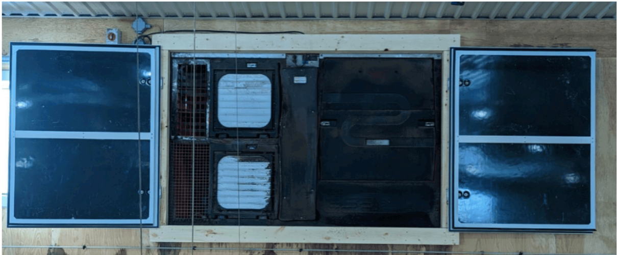
Figure 35 Winter covers installed, open position
